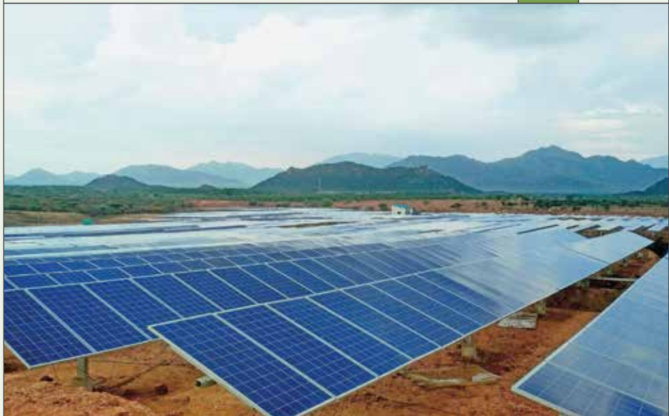
50 MWp Solar Tracker Plant, Theni, Tamil Nadu
