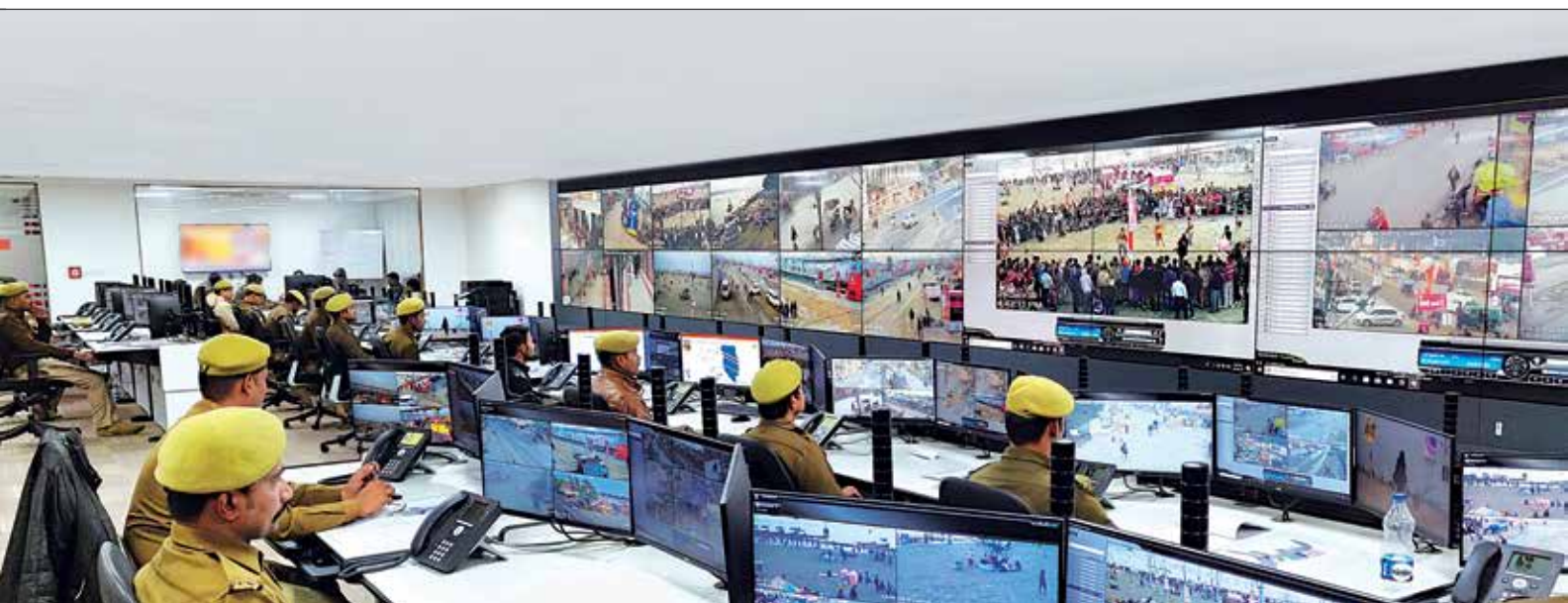
Command and Control Centre, Prayagraj Smart City
