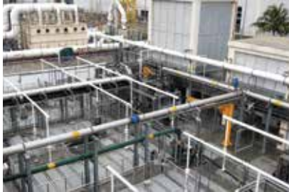
▲ Changi Wastewater Reclamation Plant
