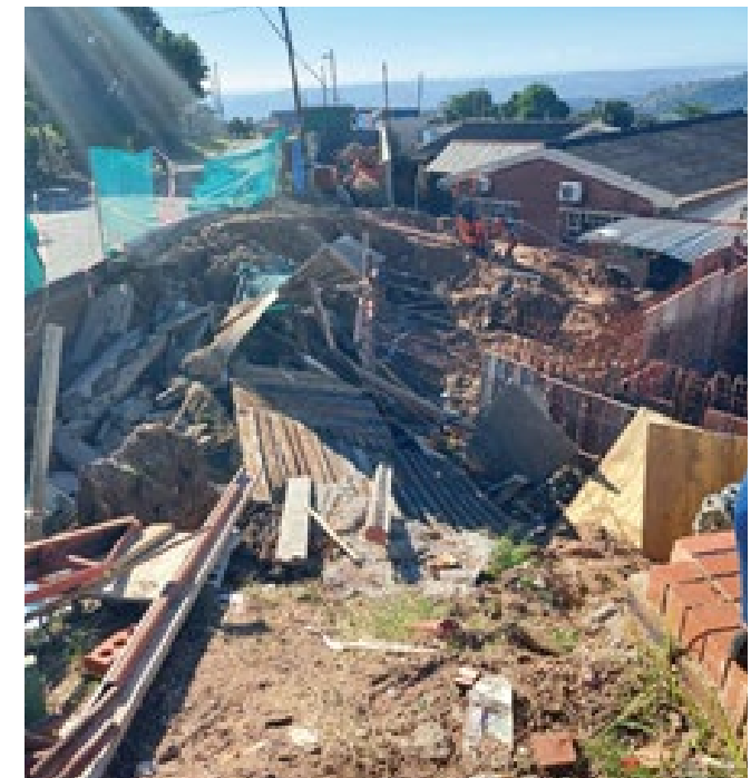
Newtown A Clinic in Inanda was severely damaged by floods in April 2022.
