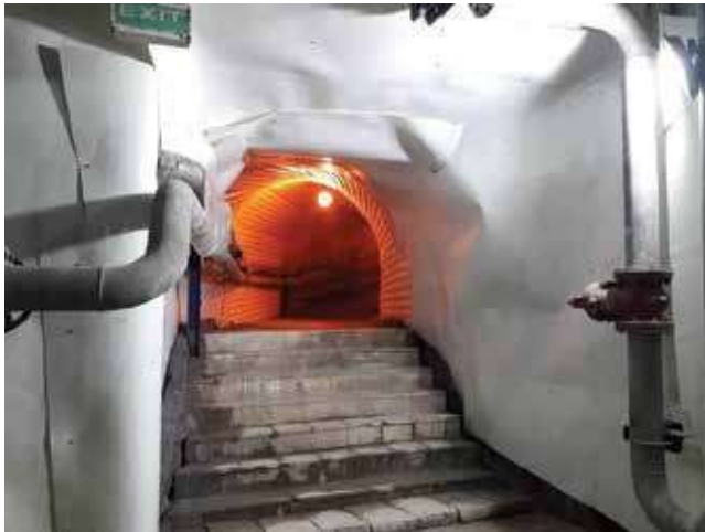
Seepage Management at Transformer Hall access tunnel.
