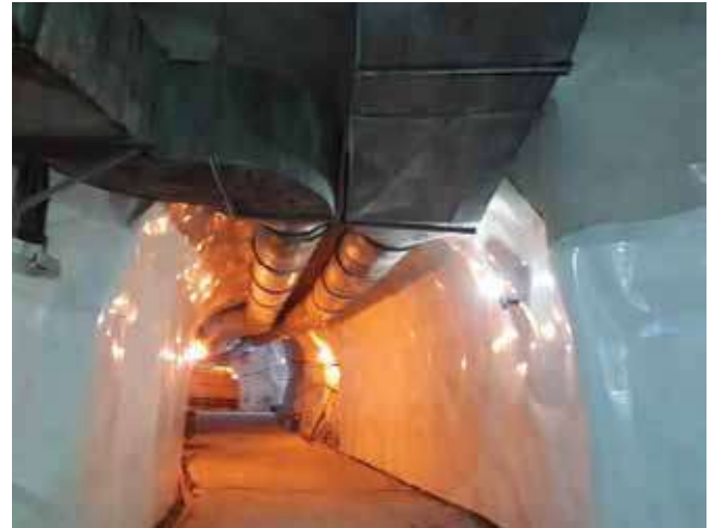
Seepage Management at Machine Hall access tunnel.
